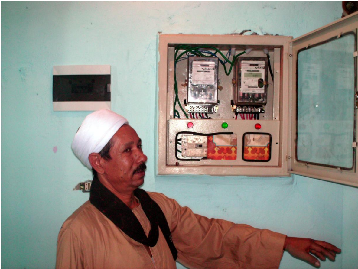
Foto 7.1: Mr. Bushra Yaakoub Salih proudly shows the upgraded power sources with the electric metre and the fuse boxes. Notice also the newly-plastered and painted walls. Oct. 30 th , 2009
